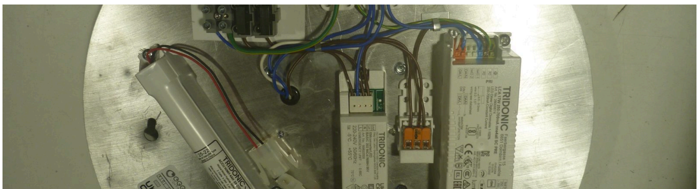
The gear tray as built: Tridonic driver and LED module, emergency converter and battery. Power and power factor were measured on 100% of units.
